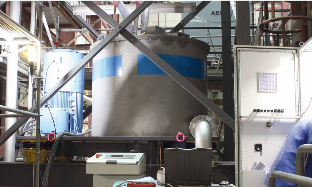
Ferrum gypsum centrifuge in operation
